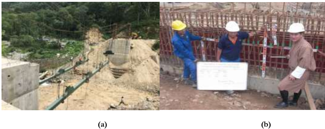
Figure 5: Comparison of working conditions between Dangdung Bridge and Dechen Bridge. (a) Workers at launching of steel girders without safety belt and PPEs. (b) Quality check/audit at Dechen Bridge with workers in proper PPEs.
