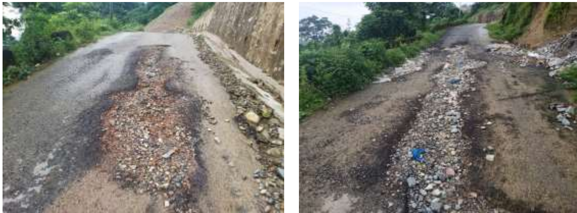
Figure 3. Post condition of pavement surface due to poor base materials
