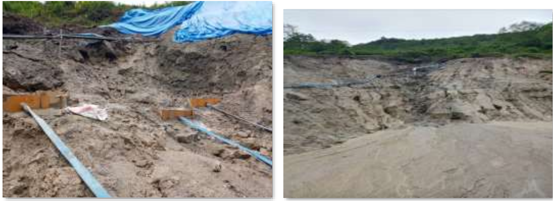
Figure 3. (a) Fan-Shaped colluviums material deposit at the base of the slope; (b) Water diversion using wooden catch basin
